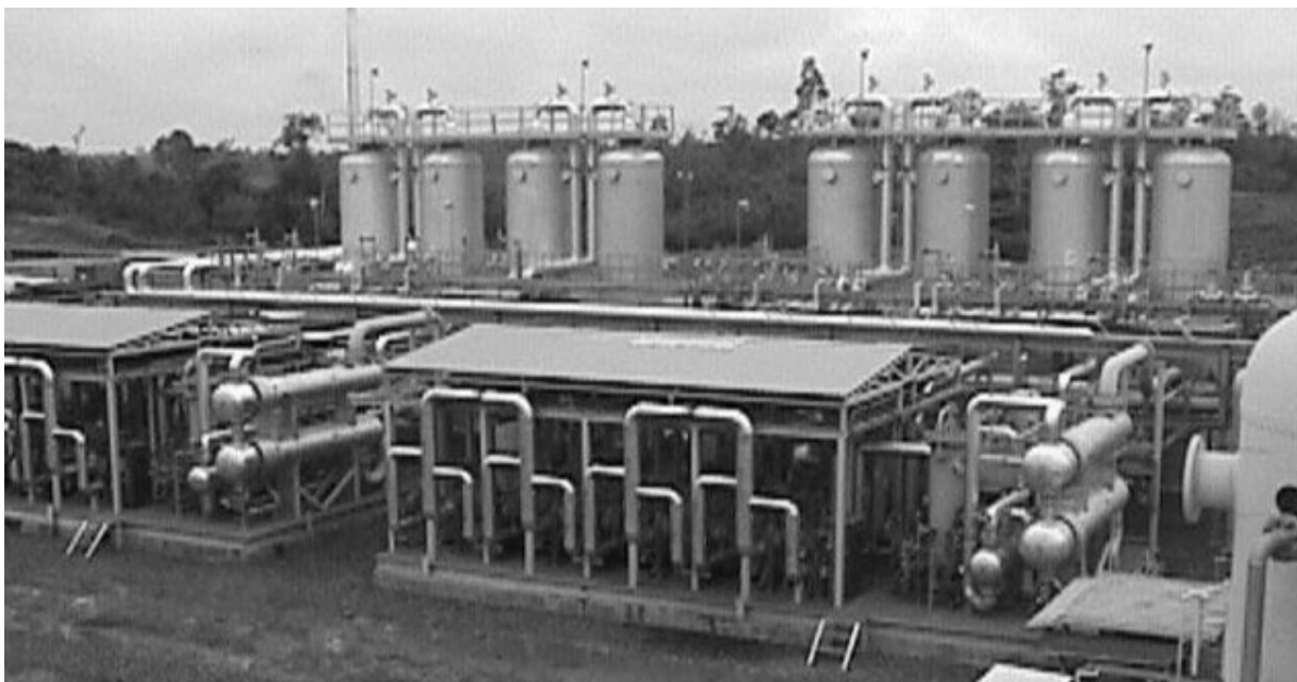
Figure 4. Engelhard Thermal Swing Adsorption Unit
